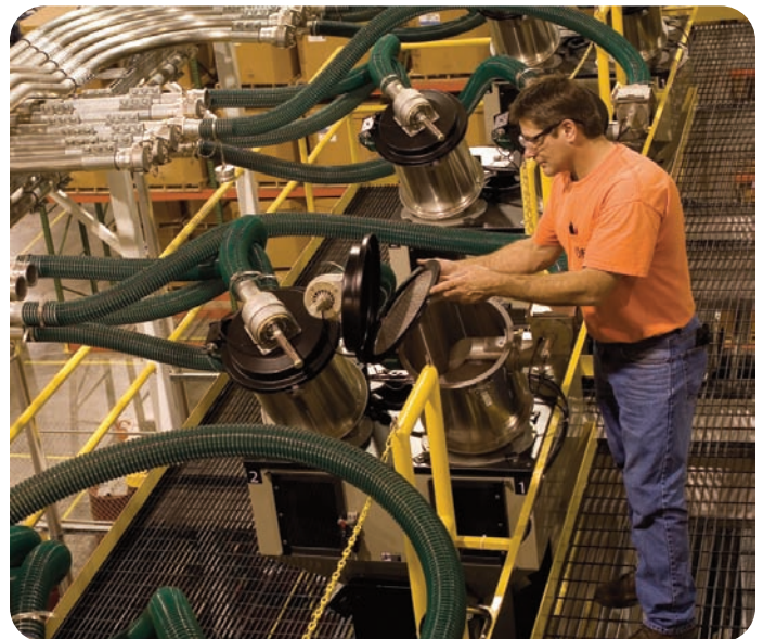
Large plants, with central material handling systems, may have dozens or even hundreds of loaders and receivers.
