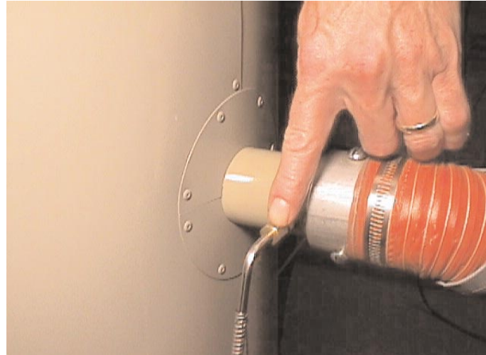
Location of the Process RTD at the Hopper inlet.
