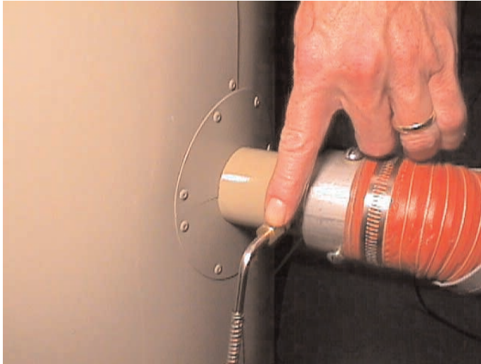
Location of the Process RTD at the Hopper
