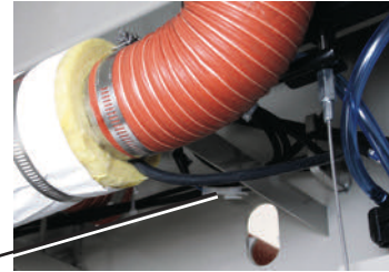
Heater Wiring Harness
