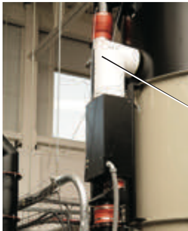
HTC Outlet to CH Hopper Inlet Connection
