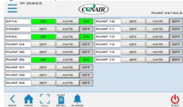
Figure 5 – Pump Details Screen
