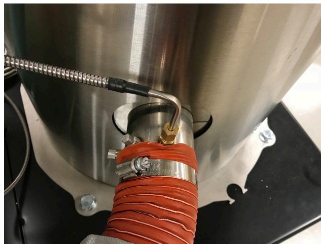
Location of the Process RTD at the Hopper inlet.
