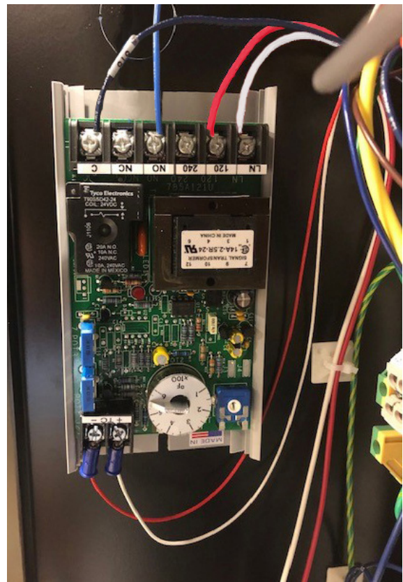
Switch with Power and Circuit Wires Installed
