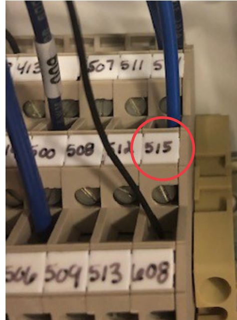
Wire 515 in Panel
