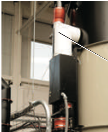
HTC Outlet to CH Hopper Inlet Connection
