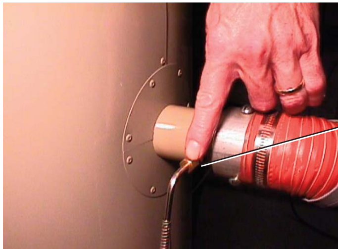
Typical location of the Process RTD at the hopper inlet.
