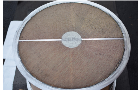
Example of a Desiccant Rotor with More Than 15% Blockage
