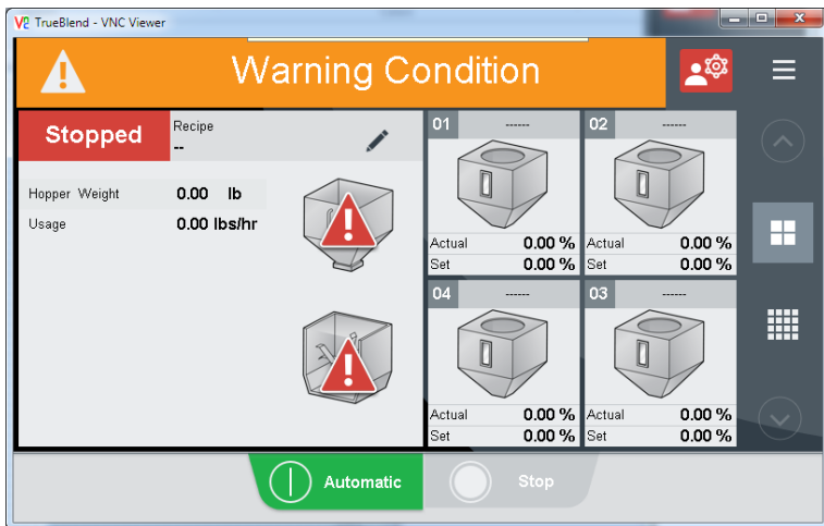
Figure 10: TrueBlend – Warning Alarm
