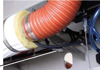
Heater Wiring Harness
