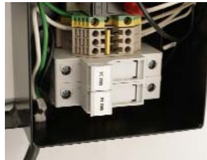
Fuses - in service
