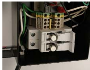
Fuse blocks open for service.
